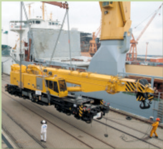
The crane is carefully lifted off the track at the Bremerhaven fruit terminal ...
